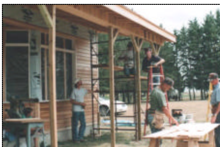
A group of Boys is working on the One Room Country School Museum Building completing the porch area. They are hopeful that they will be able to get the walkway completed so visitors can easily get from the One Room Country School to the Museum. Working on the porch are from the left and around are David Hoffman , Augusta, GA, Byron Arnold , Unionville, MI, Norm Parker , Cass City, MI, Bob Hirn , Cass City, MI and Ron Hoffman , Bad Axe, MI.
