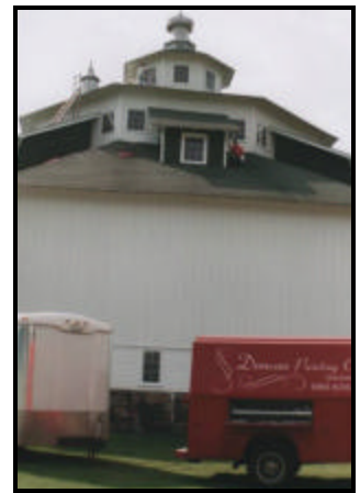
Painters from Duncan Painting are finishing off the windows on the dormers and cupola. Look closely and you will see them painting away. They look so small dwarfed by the immense size of this structure.
