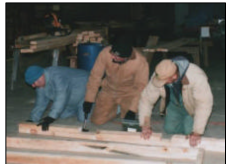
Some of the boys are pictured in the arena of the Barn constructing the walls of the Blacksmith Shop. When the weather breaks, they will be able to move these sections to the designated location next to the Sugar Shack where the foundation was already installed this past Fall. Pictured are Jack Hill, Richard Stacer & Bob Hirn building a section.
