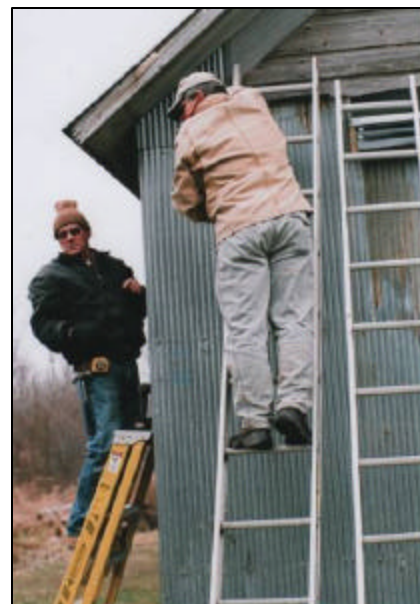
Richard Stacer and Dave Jaroch , both of Ubyly, are applying the corrugated steel sheeting to the older section of the Grain Elevator Building. First felt was fitted and stapled to the walls and then the steel was nailed in place. The building is now completely covered with the steel as the Boy's Day Out Crew has continued to work throughout the winter months.
